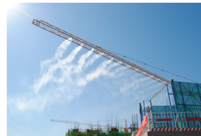
塔吊喷淋 Tower crane spraying system
