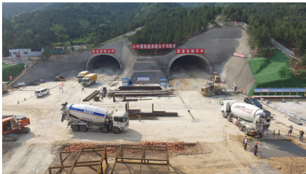
兴延高速白羊沟隧道施工 Construction site of Baiyanggou Tunnel on Xingyan Expressway
