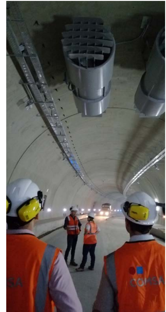
Intelligent Traffic Systems (ITS) in the Bogotá - Villavicencio Corridor (Colombia)
