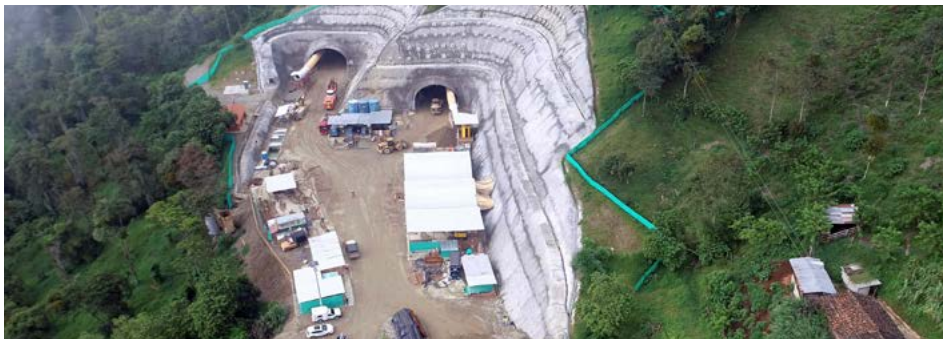
Construction of the Amagá Tunnel of the Pacific Connection Highway 1, Antioquia (Colombia)
