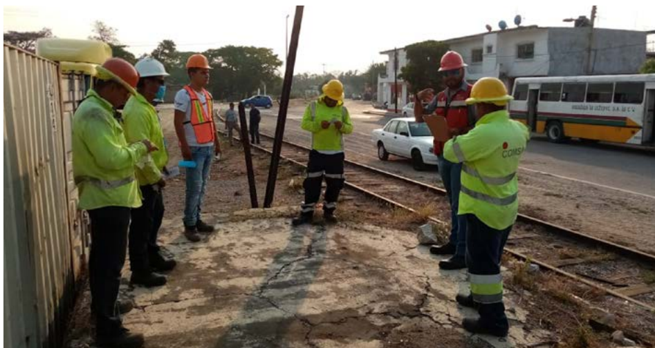
Metro Maintenance Line A (México)
