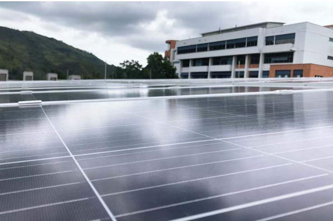
Building L solar energy, Bucaramanga Campus
