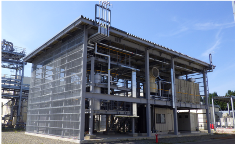
CO 2 Methanation Test Facility
