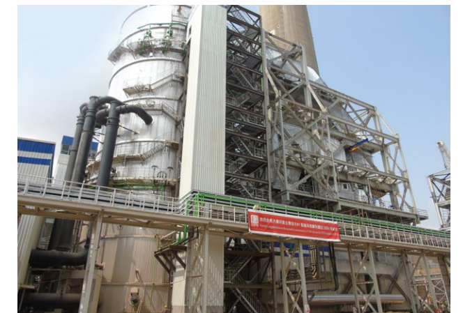
▲ The desulfurization system for No. 1 generating unit of Datang India Cuddalore Coal-fired Power Plant successfully completes trial operation.
