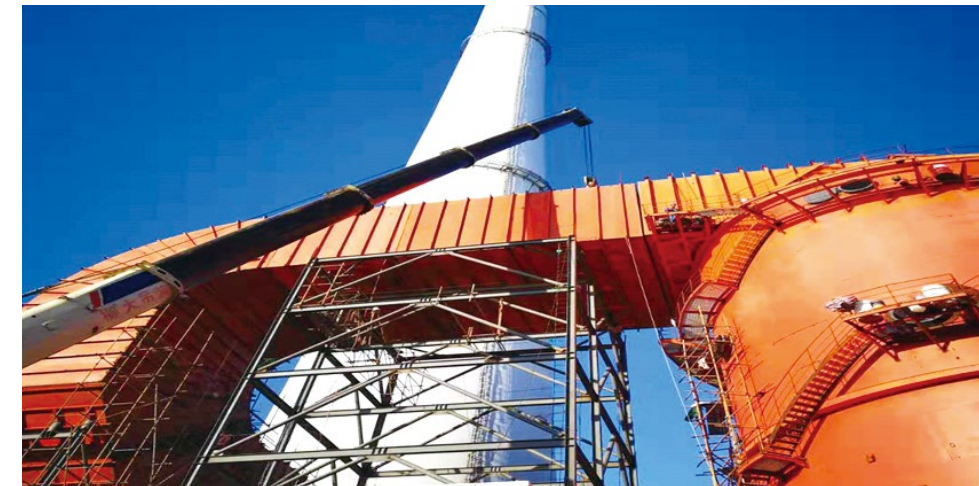
▲ Ultra-Low Emission Transformation Project of the No. 3 Generating Unit of Datang Guiguan Heshan Electric Power Co., Ltd.
