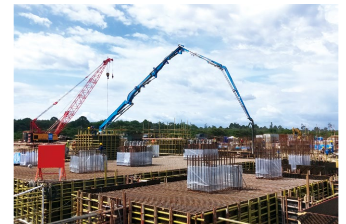
▲ Construction site of the Meulaboh 2x 225MW coal-fired power generation project, Indonesia
