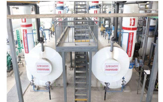
▲ On December 6, the Phase 2 Flexible Renovation Project of No. 1 and No. 2 Thermal Power Generating Units of Datang Harbin No. 1 Thermal Power Plant were successfully put into operation. As an electrode direct heating boiler coupling project, it has the largest single unit capacity and total installed capacity in China, and the thermal efficiency could reach 99.11%.
