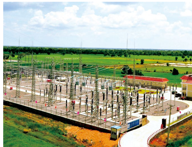
▲ The Phnom Penh to Battambang 230kV-substations project runs safely and steadily, making prominent contributions to the operation of local power grid and power supply.
