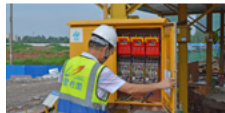
Checking safety problems
