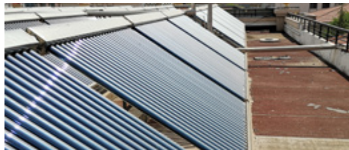
Country Garden Hotels Solar Water Heating System
