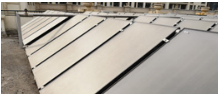
Country Garden Hotels Solar Water Heating System
