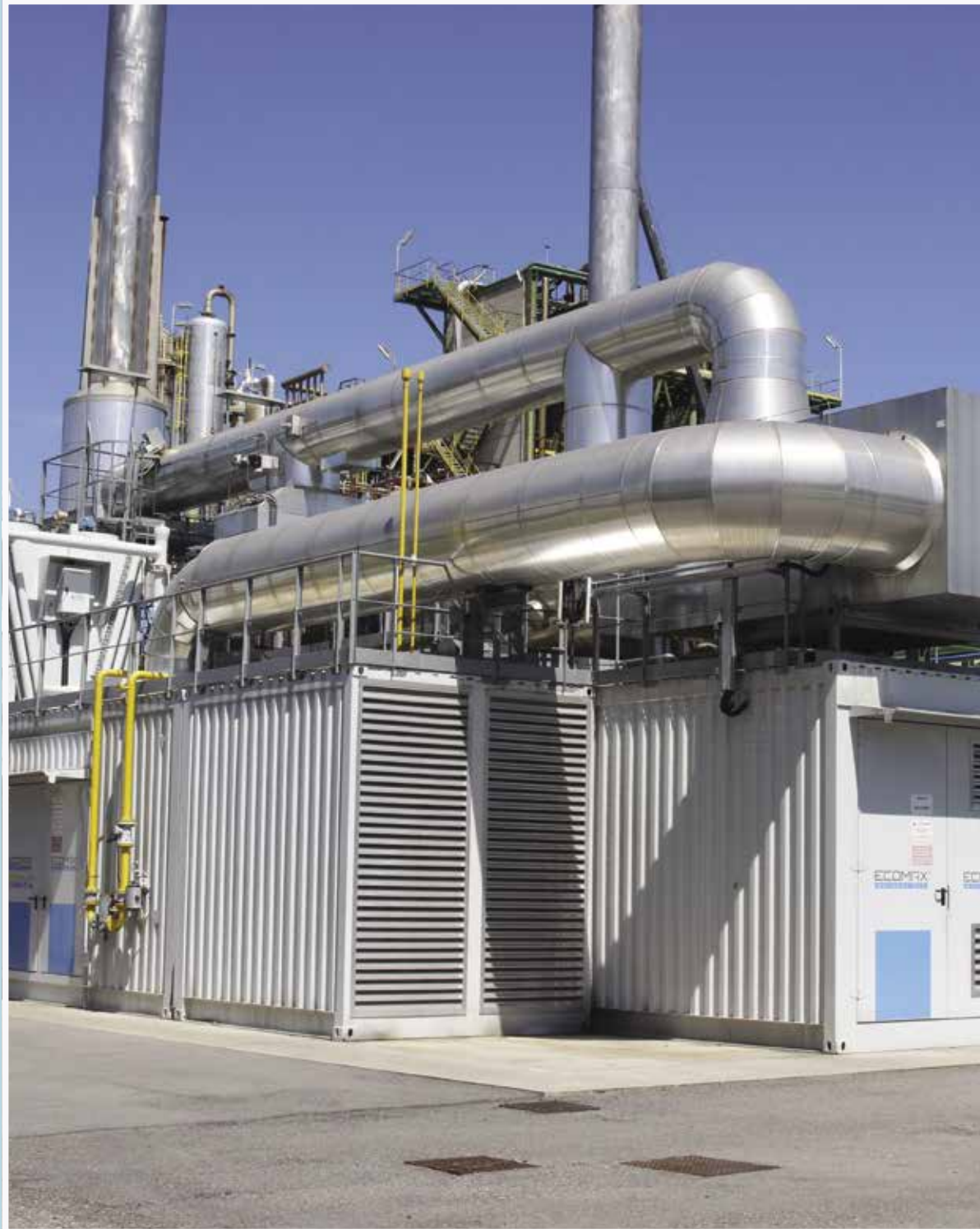
The co-generation plant at Polynt Reichhold's Scanzorosciate, Italy site.
