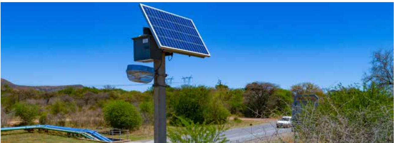
Solar-powered street lamp at BRPM
