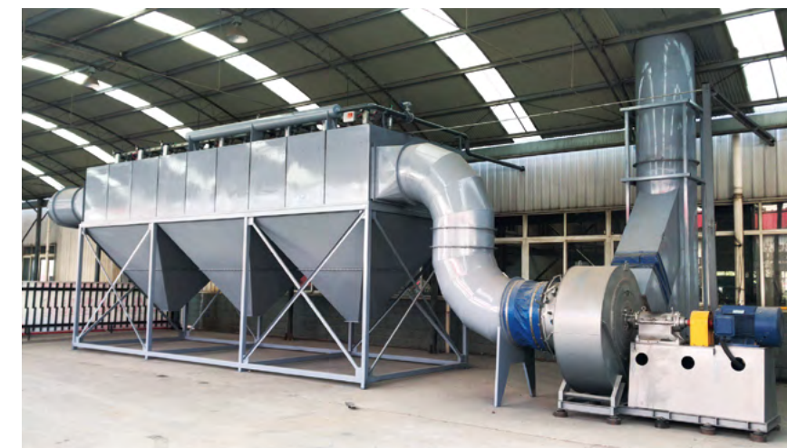
◆ Smoke treatment device improved by YTO
