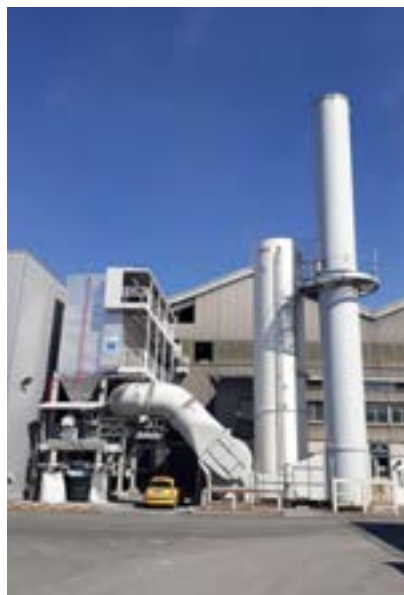
The Issoire plant's project is expected to recuperate heat from the furnace exhaust fumes to provide a new source of heat for municipal facilities
