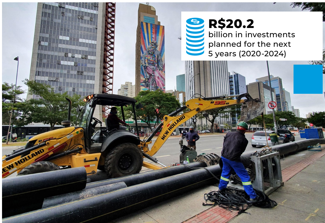
Expansion of the sanitary infrastructure of the Novo Rio Pinheiros program, on Avenida Faria Lima, in São Paulo
