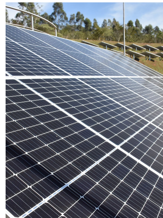
Sewage treatment plant in Mogi Mirim with a photovoltaic power generation system, installed in partnership with SESAMM (Mogi Mirim Sanitation Services)
