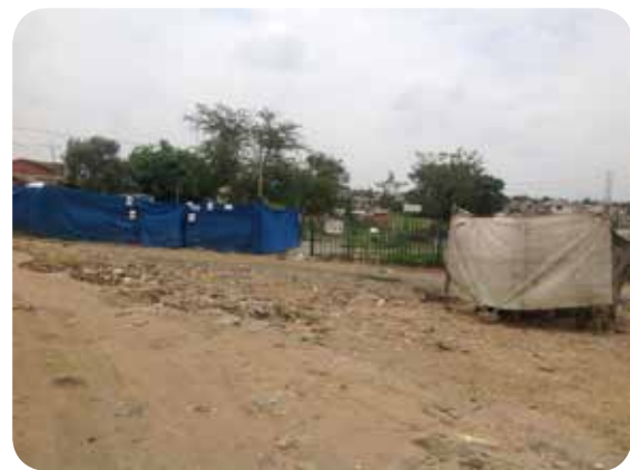
Figure 10: Site after clearance and a trench for one of the bioswales on Ward 113 site.
