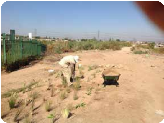
Figure 18: One of the community workers employed for the post completion maintenance clearing the swale from sedimentation after a rain event.
