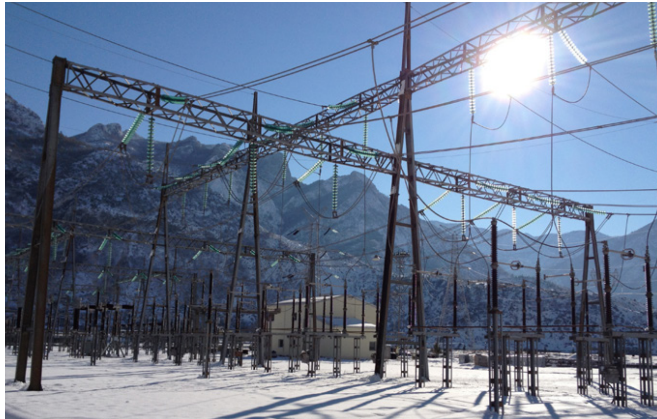
220/6 kV switchyard Koman in Albania, fully revitalised by KONČAR
