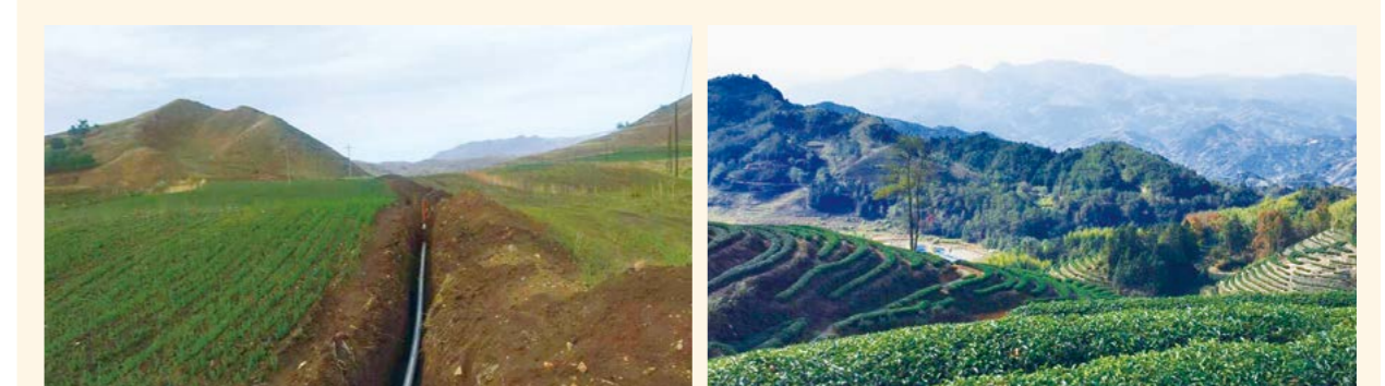
A water conservancy project was constructed in Daluhao Village, Wuchuan County, Inner Mongolia Autonomous Region to meet the water demand for local crop growth and provide long-term guarantees for farmland cultivation
