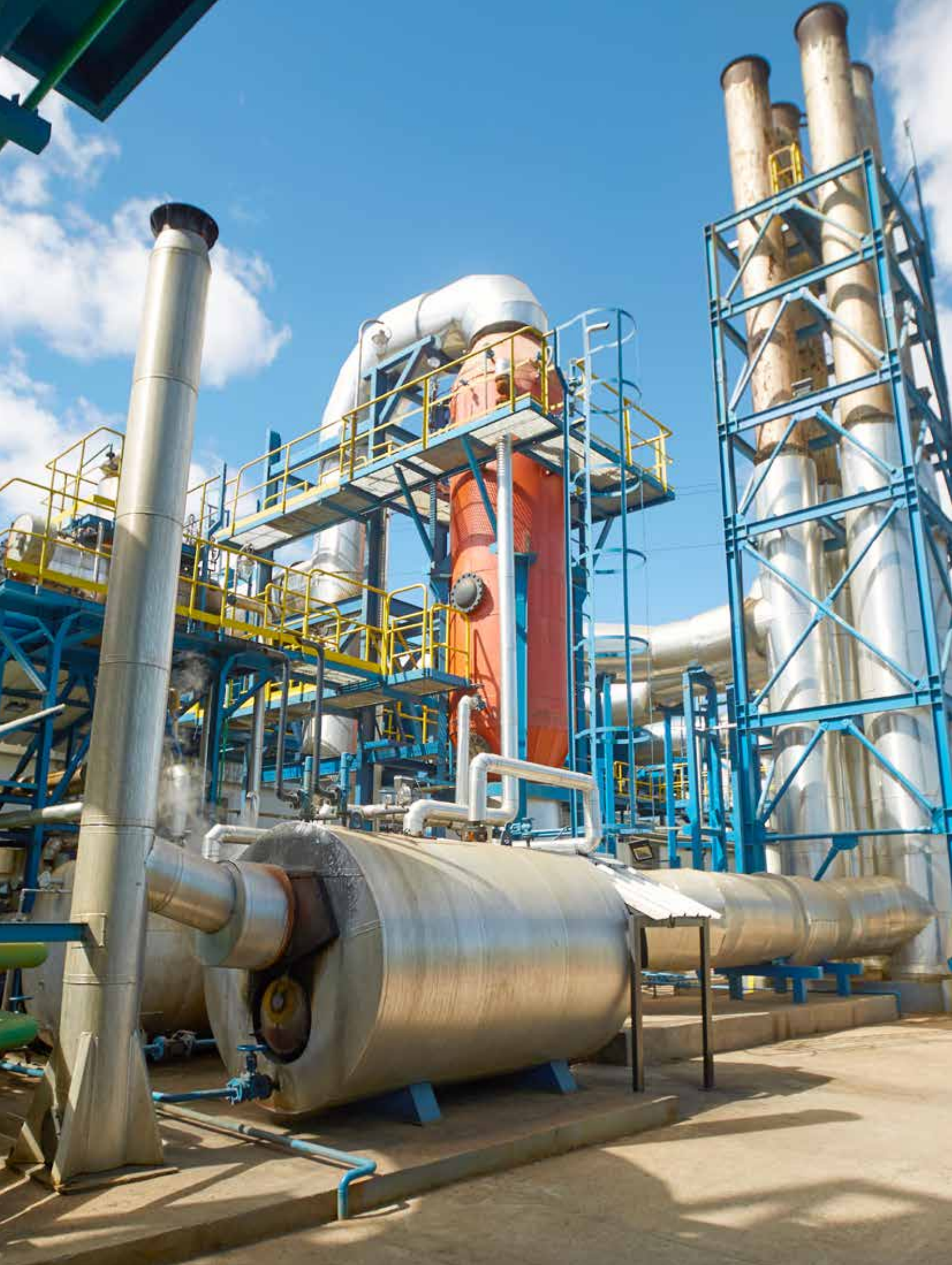
Madagascar Heavy Fuel Oil Power Plant
