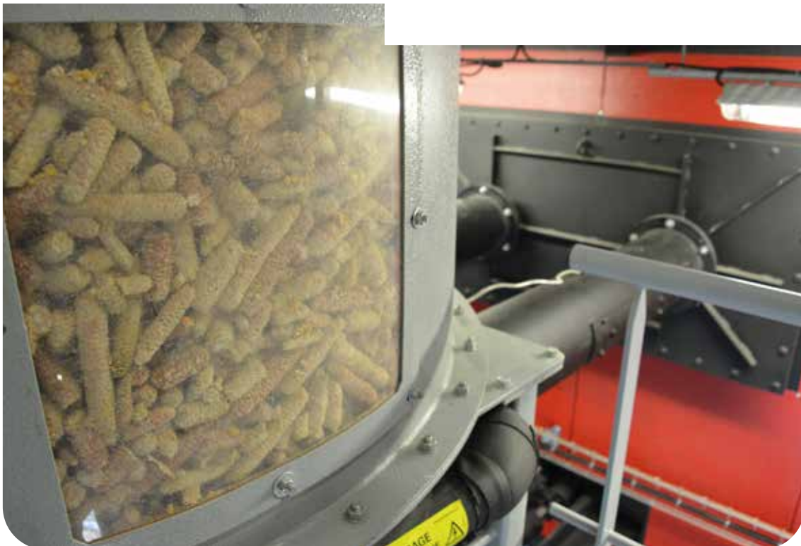
Limagrain Ingredients: a boiler installed on the Ennezat site (France) producing energy from corn cobs from Limagrain Coop seed production.
