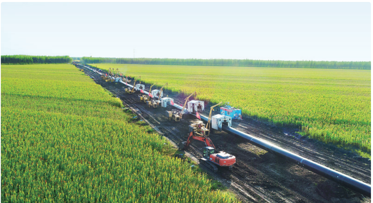
Site of the China-Russia East Natural Gas Pipeline
