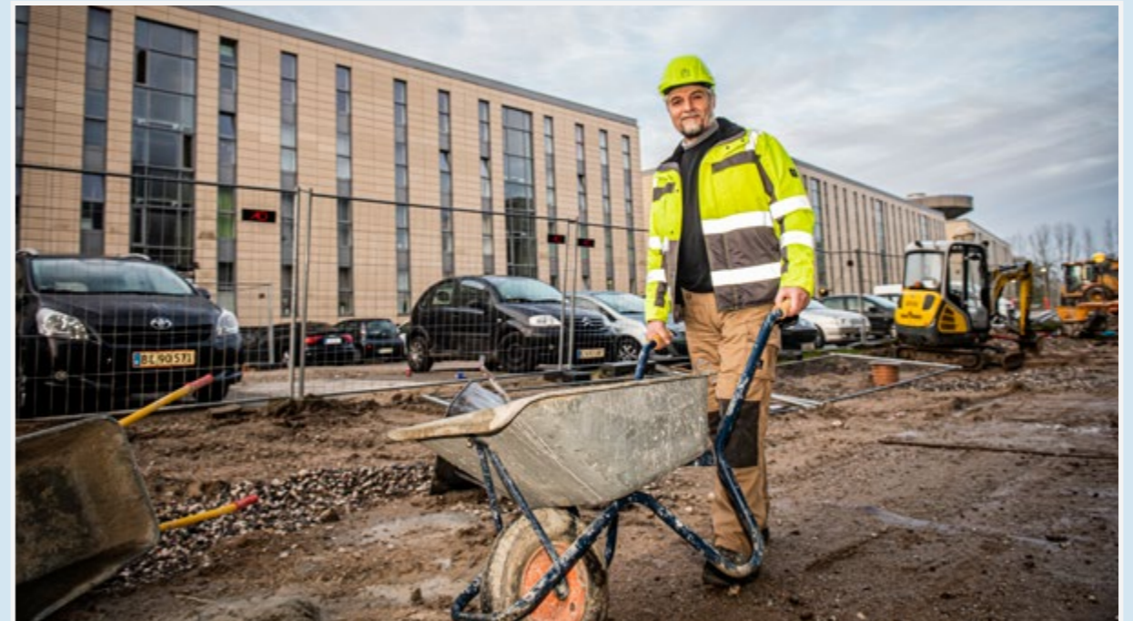
Osman carrying out safety and security renovation at Bispehaven, Aarhus, for Enemærke & Petersen under a social clause.
