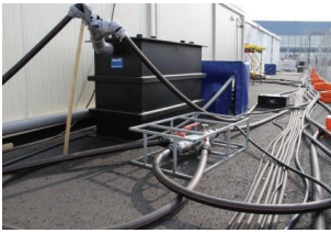
Temporary water supply and drainage system
