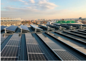
Solar PV system & Solar heat thermal system Musashino Forest Sport Plaza
