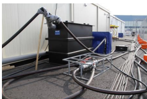
Temporary water supply and drainage system
