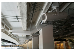
Air flow generating fan © Japan Sport Council
