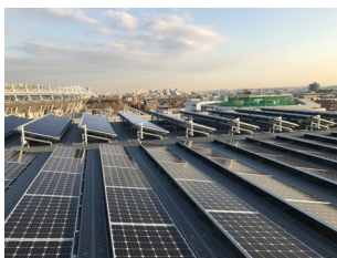
Solar thermal system and solar panels (Musashino Forest Sport Plaza) © TMG
