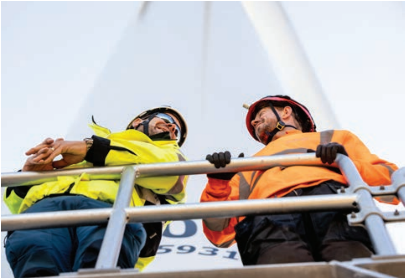
Cooperation in the supply chain during the construction of Orrberget wind farm (33 MW) in Sweden. Photo: Joakim Lagercrantz
