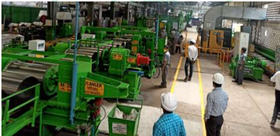
Fume Extraction System at IP – Silvassa
