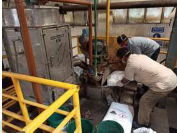
Dust collector at the Lithium Hydroxide dosing area, G&L – Manali
