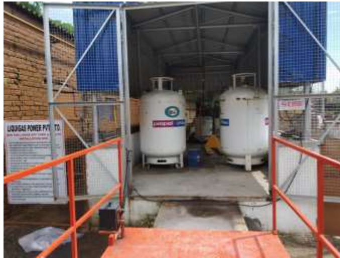
LPG being used as fuel in baking oven at IP – Kolkata
