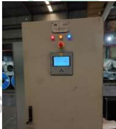
Active Harmonics Filters at auto welder, IP - Taloja
