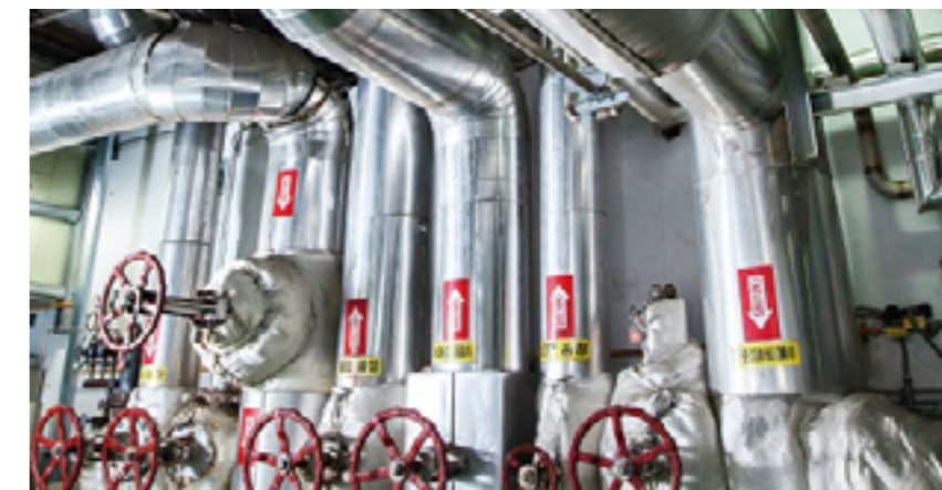
Steam pipelines for recycling external waste heat
