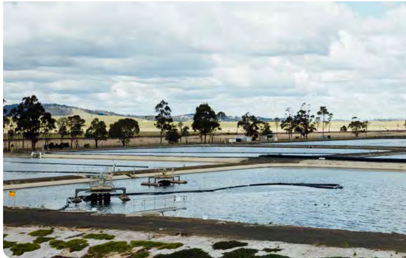
IMAGE: Recycled water lagoons at the Wallan Sewage Treatment plant
