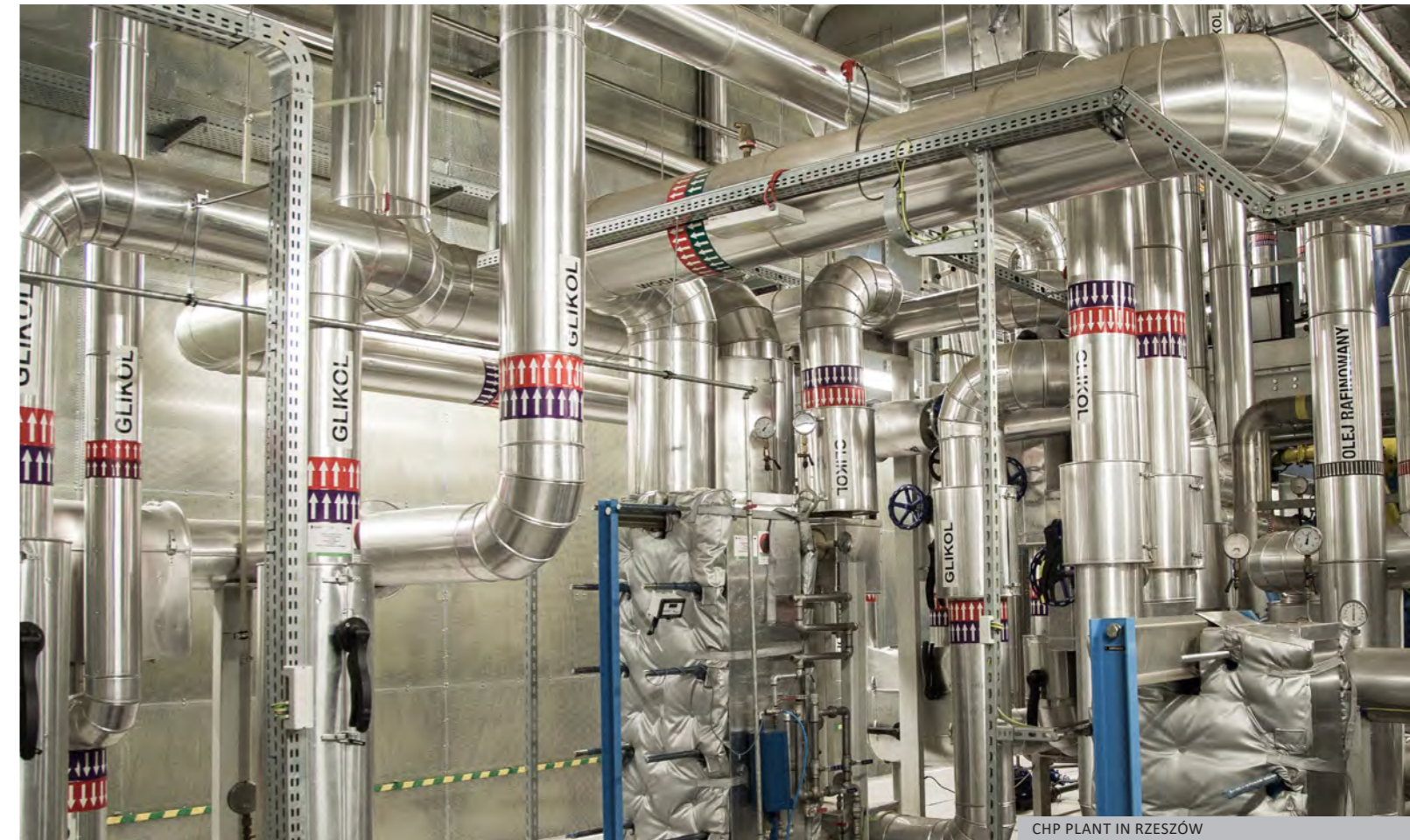
CHP PLANT IN RZESZÓW
