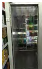
A curtain installed in a walk-in refrigerator
