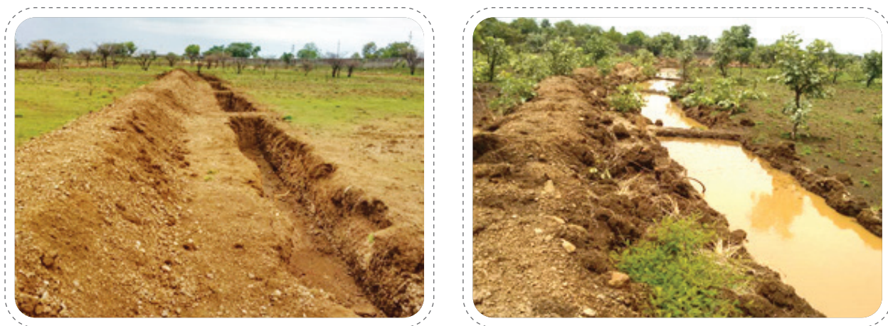
Trench Cum Bund after excavation and filled in Trenches during the monsoon. All this water captured would have gone out of the site as run off
