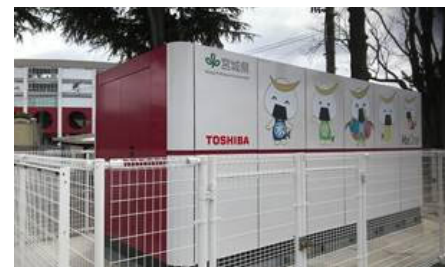
H2One™ installed at Miyagi Prefecture
