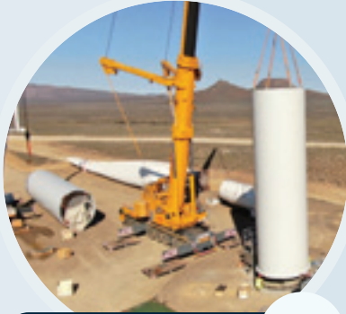
Perdekraal East Wind Farm 110 MW
