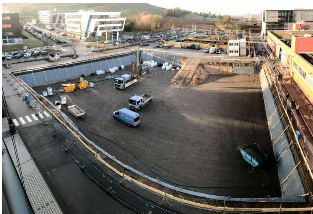
In 2019, construction of and geothermal boring for the new office building at the headquarters began. One of the 42 boreholes.
