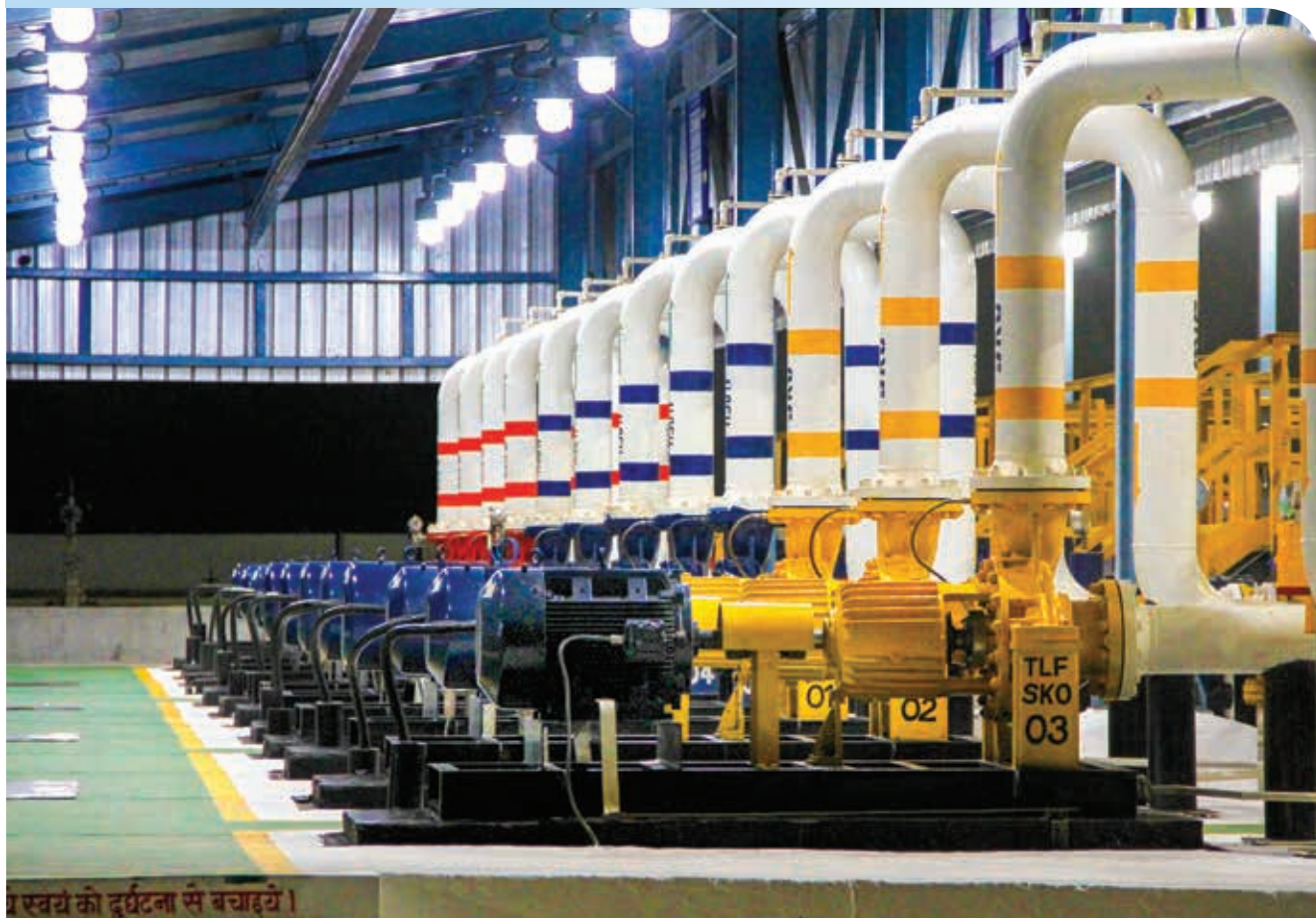
VFDs for product pumps and LED lighting in sheds for energy conservation
