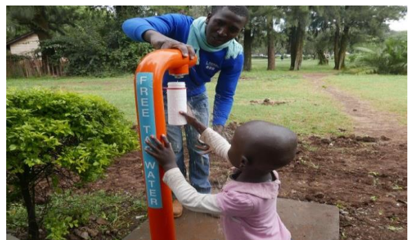
Uhuru Park Public Drinking Water Station
