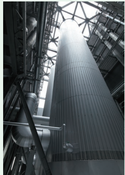
Cold water vertical thermal storage tank at Tokyo Data Center I
