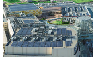
Rooftop solar panels at LaLaport KASHIWANOHA
