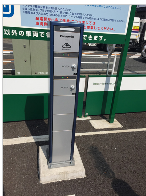
EV and PHV charging station at the Mitsui Repark Henn na Hotel Maihama Tokyo Bay Parking Lot (Urayasu City, Chiba)
