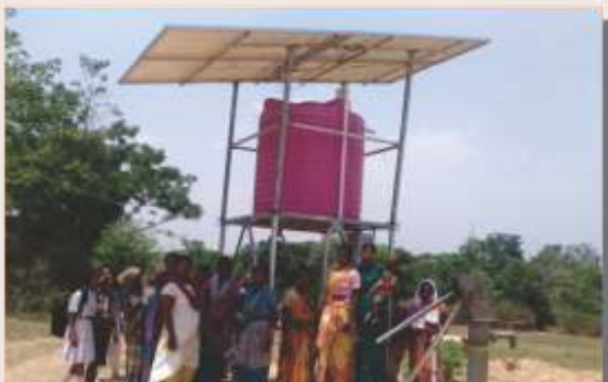
Mini Piped water supply installed from 14 th Finance Commission, Gundu village (Ranchi) July 2018
