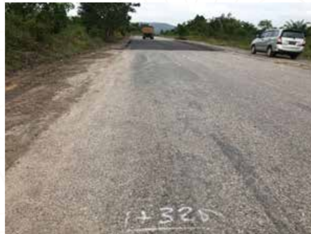
Soewandi Street Repair (overlay and patching) as the connecting road between Soekarno-Hatta Street and Sangatta-Bengalon Axis Road
