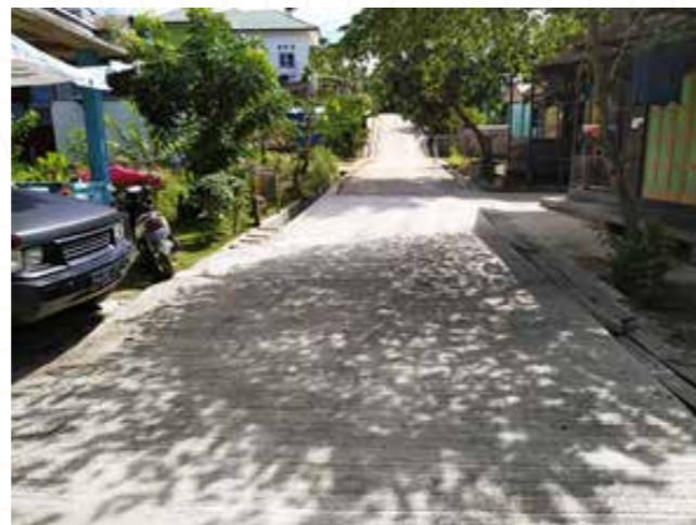
Cementing of Pelangi aisle, RT.39, Bukit Pelangi, Teluk Lingga Village, North Sangatta
