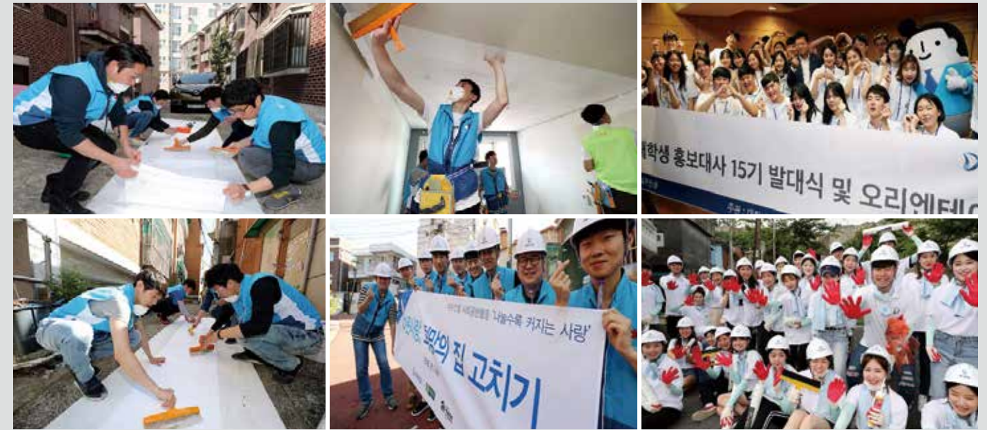
① ② ③ ④ The Building Houses with Hope Program ⑤ ⑥ "Habitat" Activities by College Student Ambassadors
