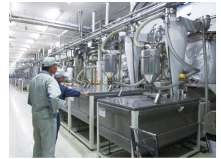
Resin drying equipment at the Xicen Plant in China
