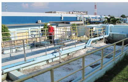
Cebu Mitsumi's water treatment facility
