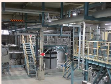
Demonstration Plant for MinerPa®
