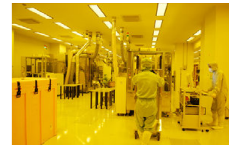
Cleanroom for photoresist manufacturing
