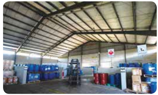
New chemical warehouse which facilitates the systematic and safe storage of chemicals
