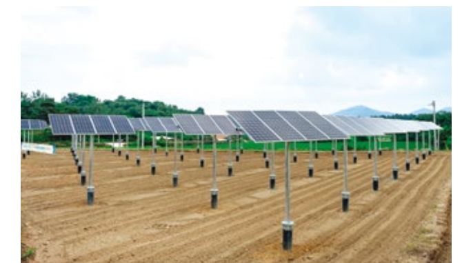
▲ Grid-connected solar photovoltaic power generating system in agricultural management. No.1
