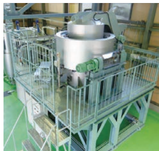
Supercritical CO 2 cleaning plant
