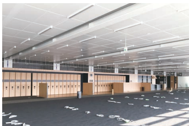
Indoor space with ceiling cooling panels
