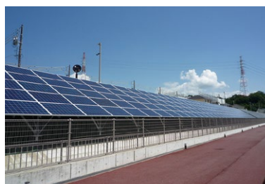
Solar power plant in Hidamari-no-Oka
