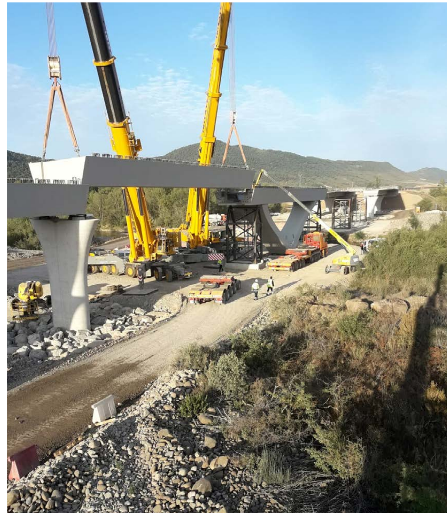
Works for the construction of the A21 Santa Cilia - Puente la Reina de Jaca Motorway, Huesca (Spain)
