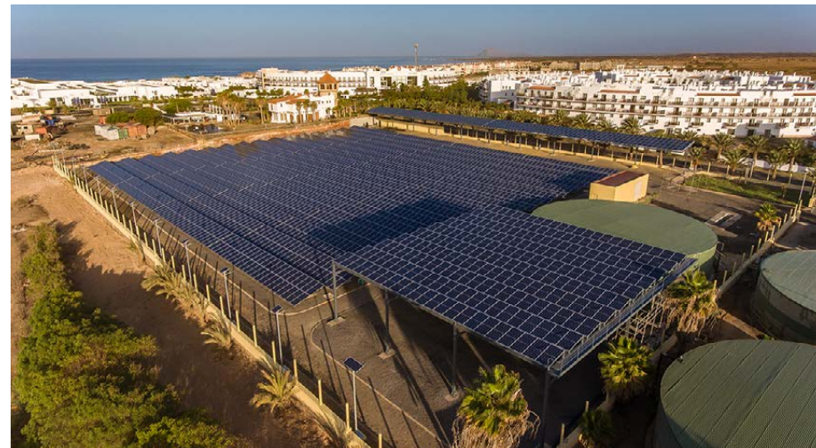
Solar plant built by TFM on Salt Island, Cape Verde (Africa)
