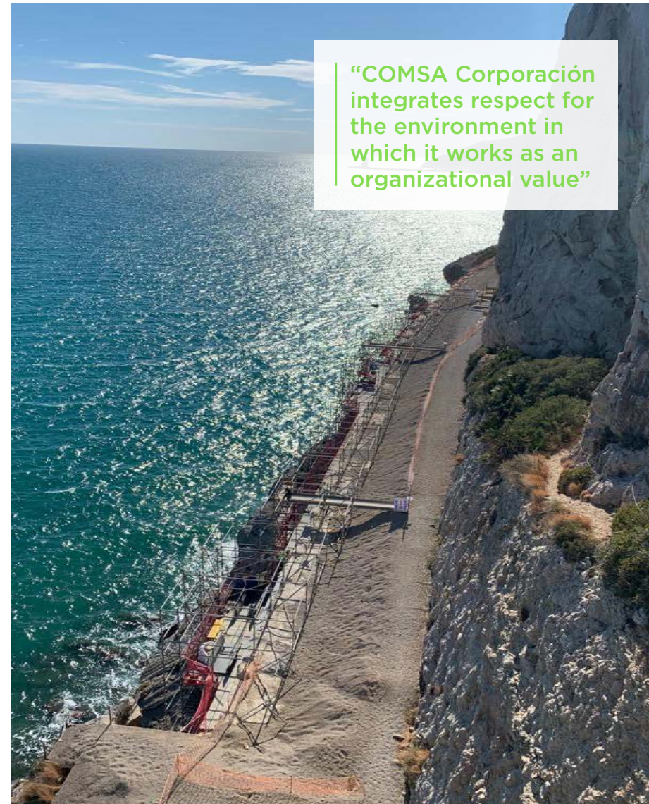
Repair work on the 98 Bis Artificial Track Tunnel for the 200 Madrid-Barcelona Sants Line (Spain)
