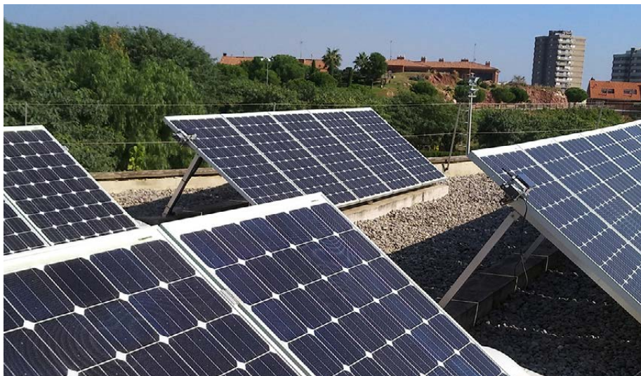
The REFER project applied to the Tirant lo Blanc library in Montgat (Spain)
