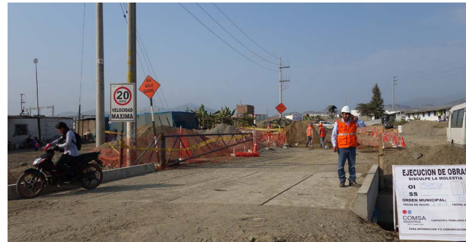
Construction of a bridge to improve mobility in the municipality of El Rosario (Peru)
