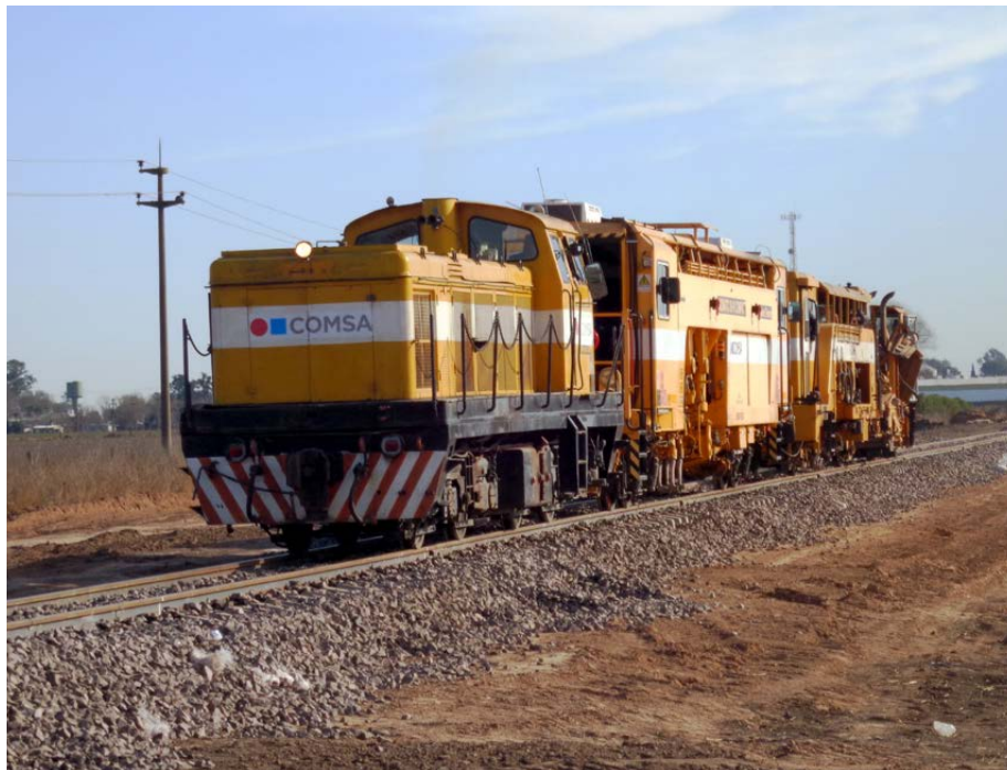
Renovation of the Monjes - Timbúes railway track section, in the province of Santa Fe (Argentina)
