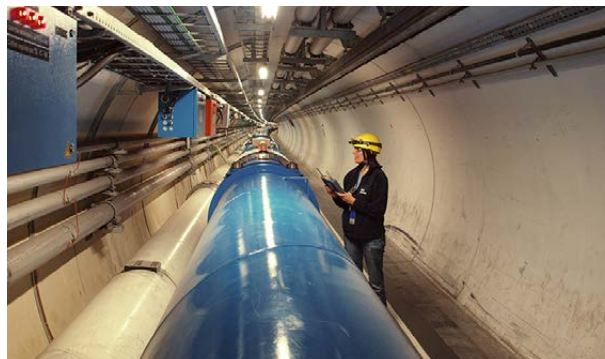
Maintenance of electrical installations at the CERN headquarters in Preveissin (France) and Meyrin (Switzerland)
