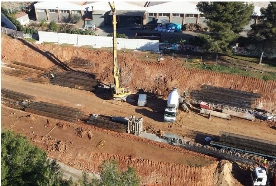
Installation of acoustic screens during the extension of the FGC underground works in Sabadell (Spain)
