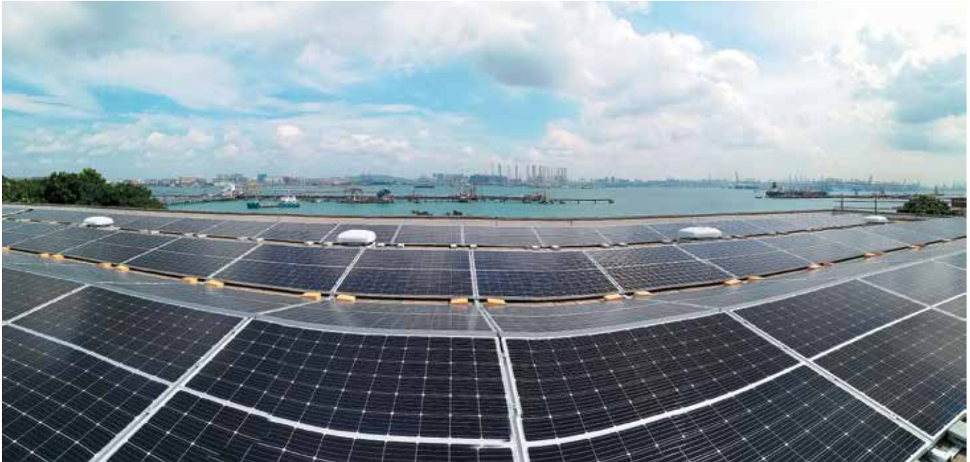
⚡ Part of the solar PV installation at YTL PowerSeraya power plant in Jurong Island, Singapore
