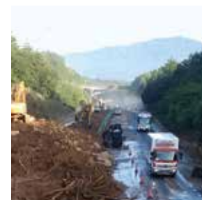
One lane is reopened after debris was removed (San-yo Expressway recovery project).
