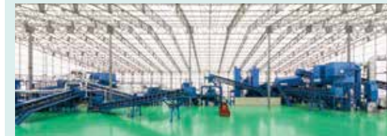
Inside the soil receiving and sorting facility
