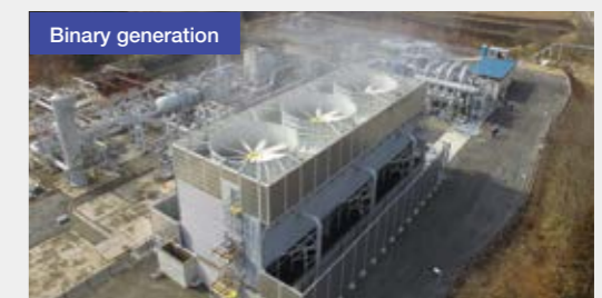
Takigami Binary Geothermal Power Station of Idemitsu Oita Geothermal Co., Ltd. (5.05 MW generation capacity, Oita Prefecture, Japan)
