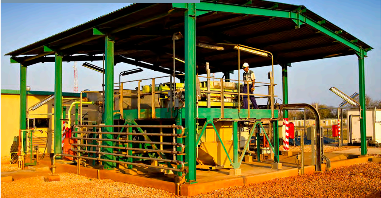
Water treatment at the Central Processing Facility, Mozambique
