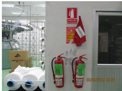
▲Fire extinguishers and emergency evacuation flags
